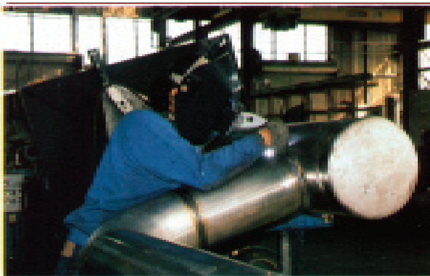
A welder attaching a piping section to a smooth-drawn tee outlet—a special feature of Alaskan prefabricated piping.
